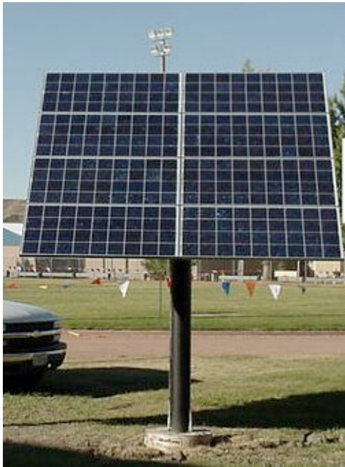
Free-standing, pole mount grid-tied PV system for school. Retrofit and Pre-Check (pre-certified) design potential, thus reducing the cost of installation.
